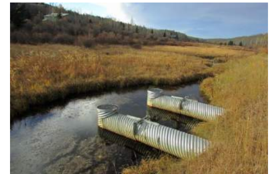
Pond leveller at Upper Fish Creek
